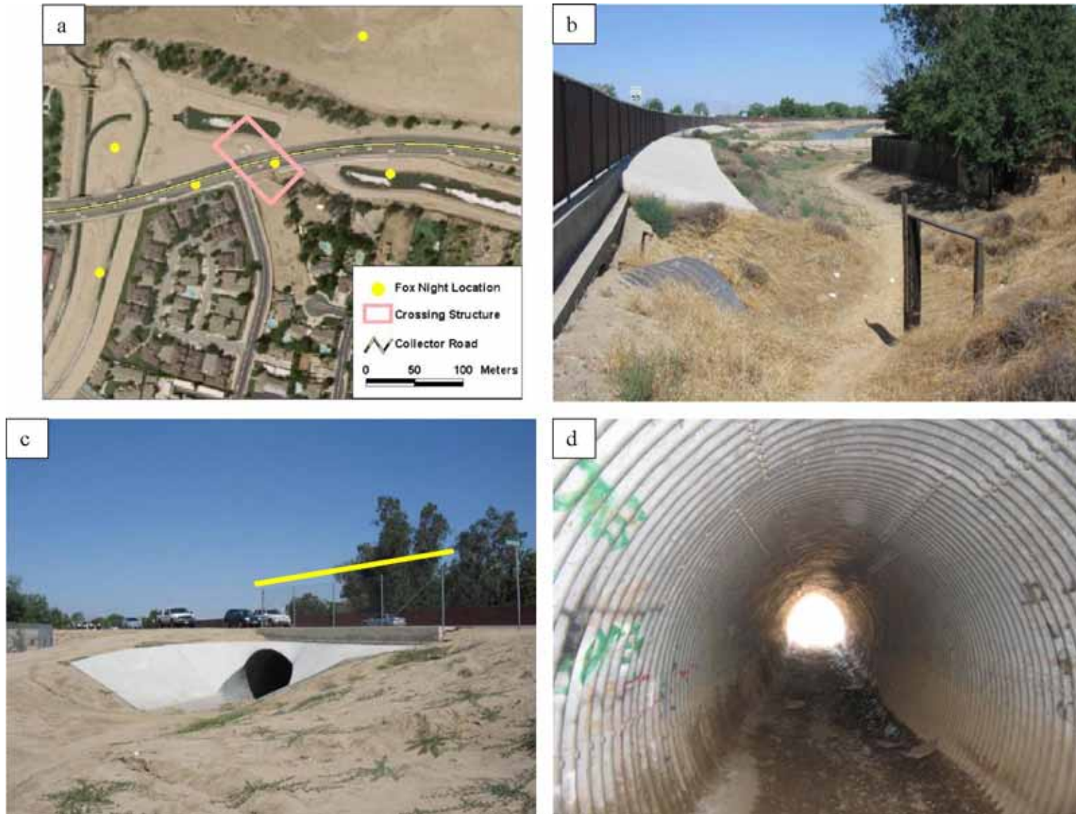
Figure 23. Truxtun Extension horse culvert, Bakersfield, CA. a) Aerial view of radio-tagged kit fox locations at horse culvert. b) View from pedestrian trail at south culvert entrance (canal in background). c) North culvert entrance. Yellow line depicts extent of fencing on north side of road. d) Culvert interior.
