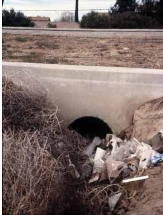
Figure 11. Drainage culvert under Highway 99 in Bakersfield, CA that was used as a den by San Joaquin kit fox.
